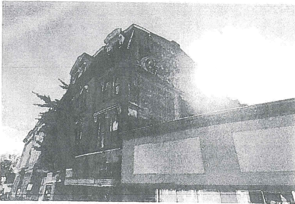
Photo #1 – Deteriorated Mansard Roof (with loose bricks) at northwest corner of Star Theater Building
